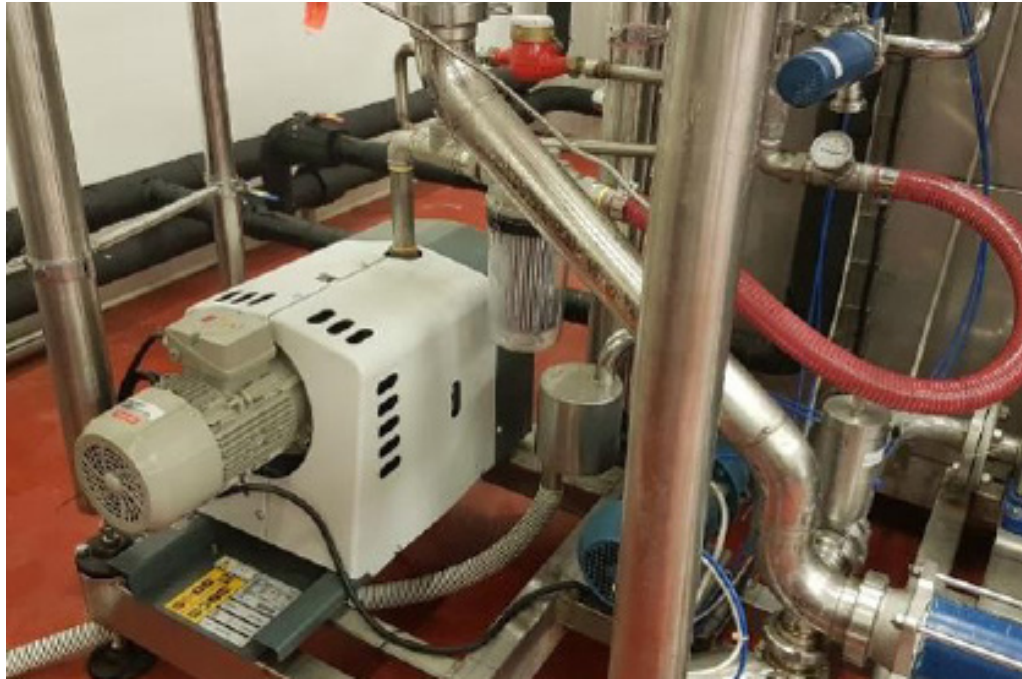
CLAWVAC installed on pasteurization system - Alain Milliat
